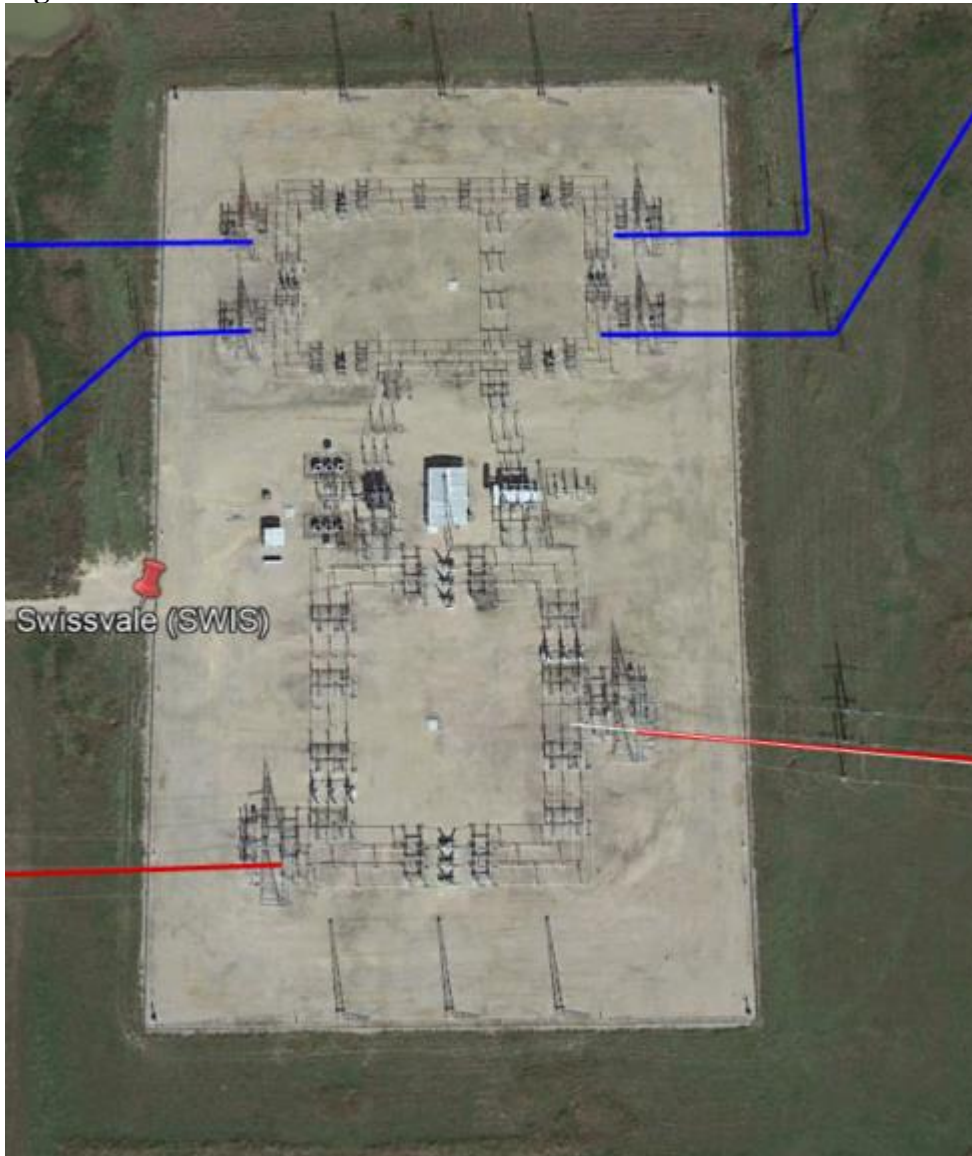
Figure 25 – Swissvale 345kV Substation
